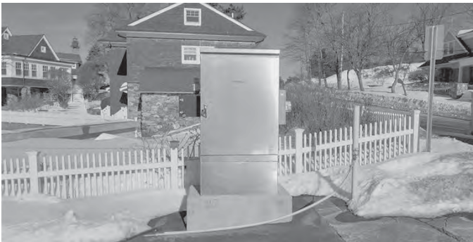
Figure 4: Nahant Street Pump Station Electrical Box
